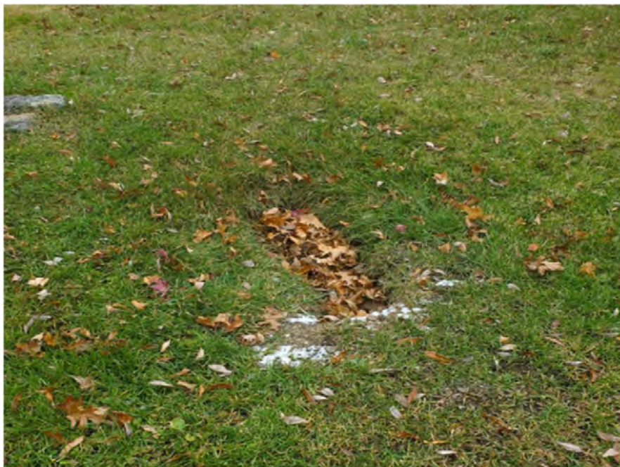
The existing condition in the backyard of 207 Laurel Street. Sinkhole in the drainage easement .
