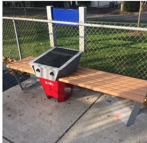
Figure 6: Solar powered phone charging bench at the Common
