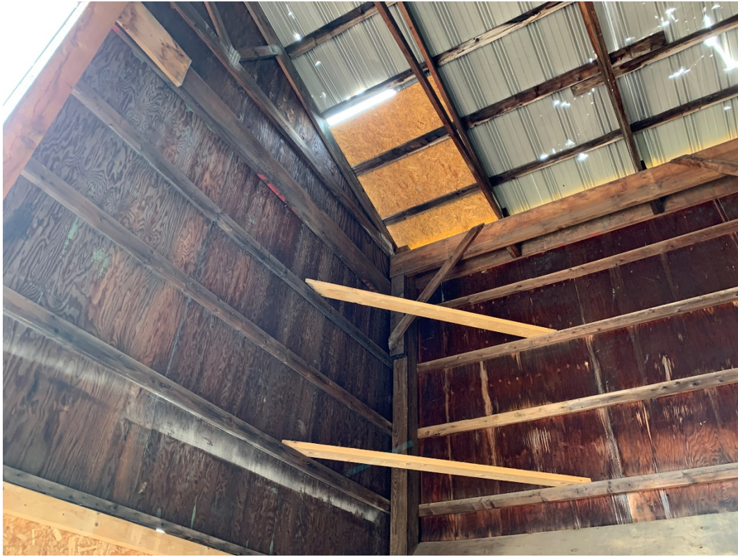
Photo 3: Holes in metal roof with plywood repair. Replaced bracing and wall panel
