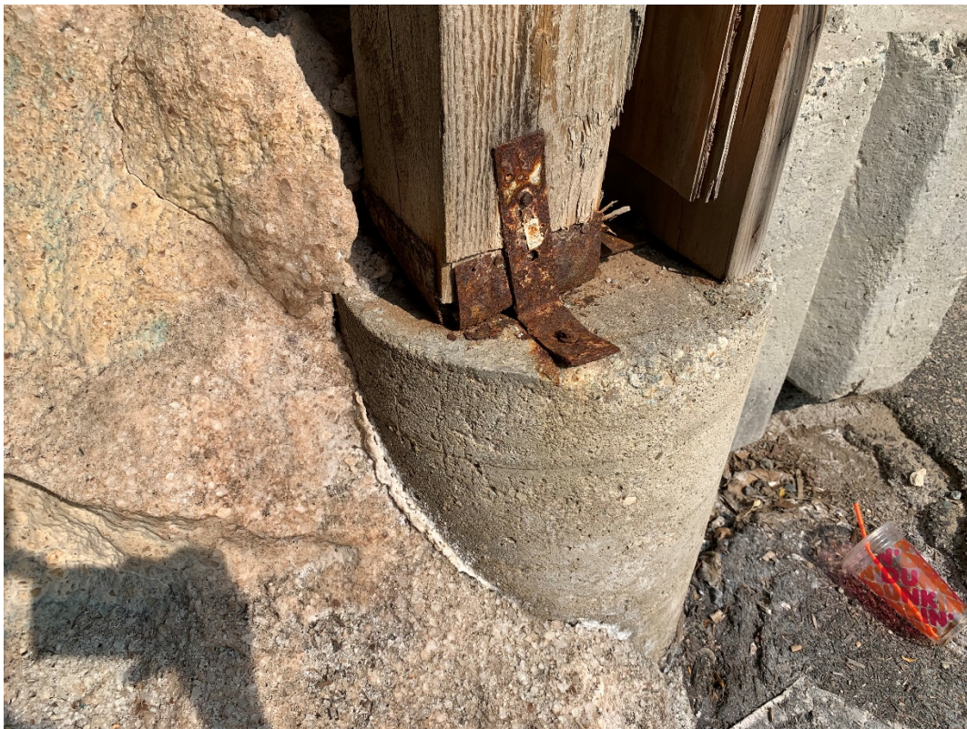
Photo 2: Corroded steel foundation connection at entrance
