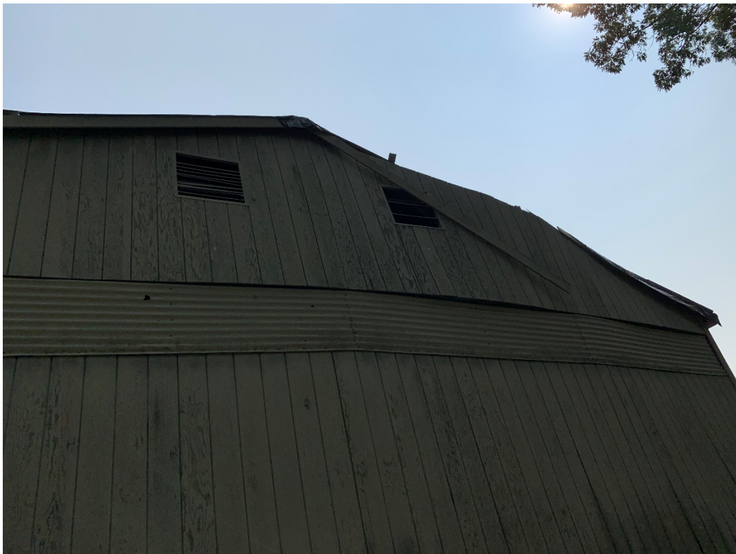
Photo 6: Damaged trim work and damaged louvers
