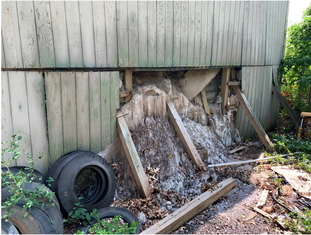
Photo 5: Failed/missing back wall panel
