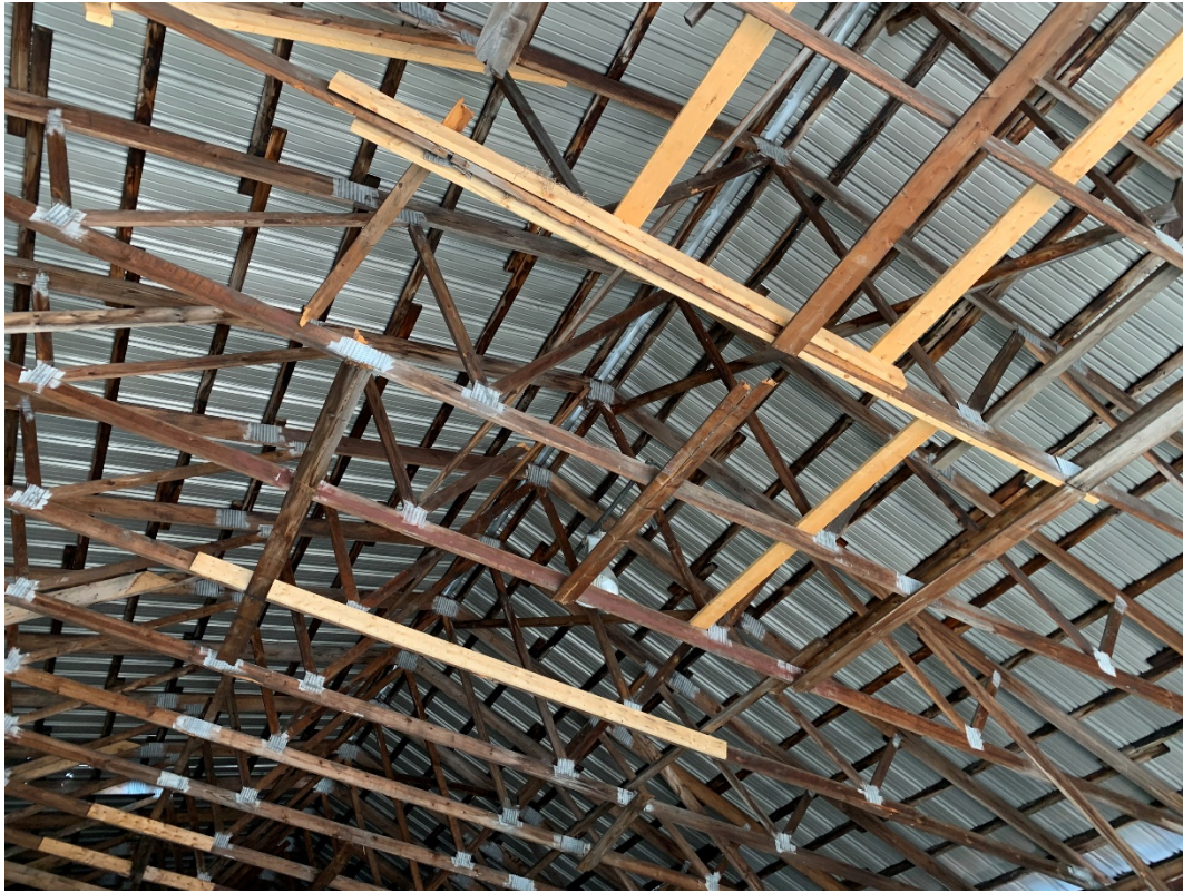
Photo 1: Sistered/damaged timber trusses and bracing
